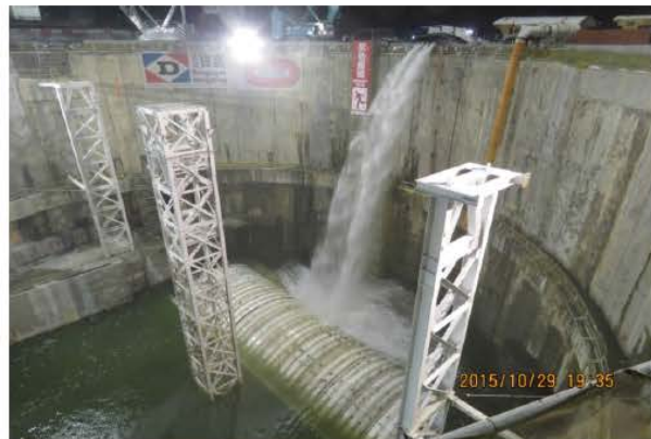
Shaft Flooding for S880 B/O
