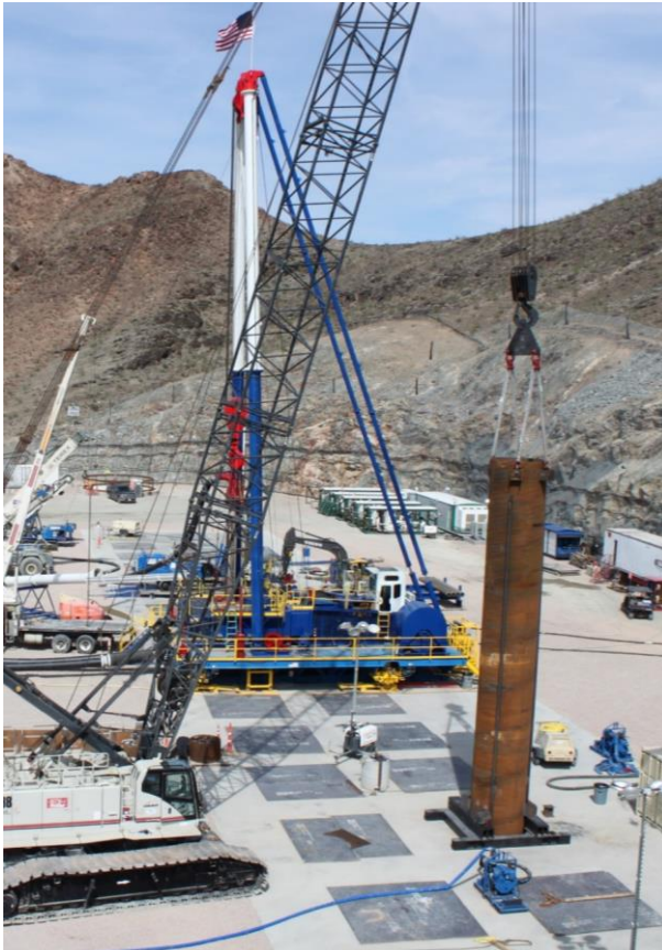
Well Casing (72" dia, 1" thick)
