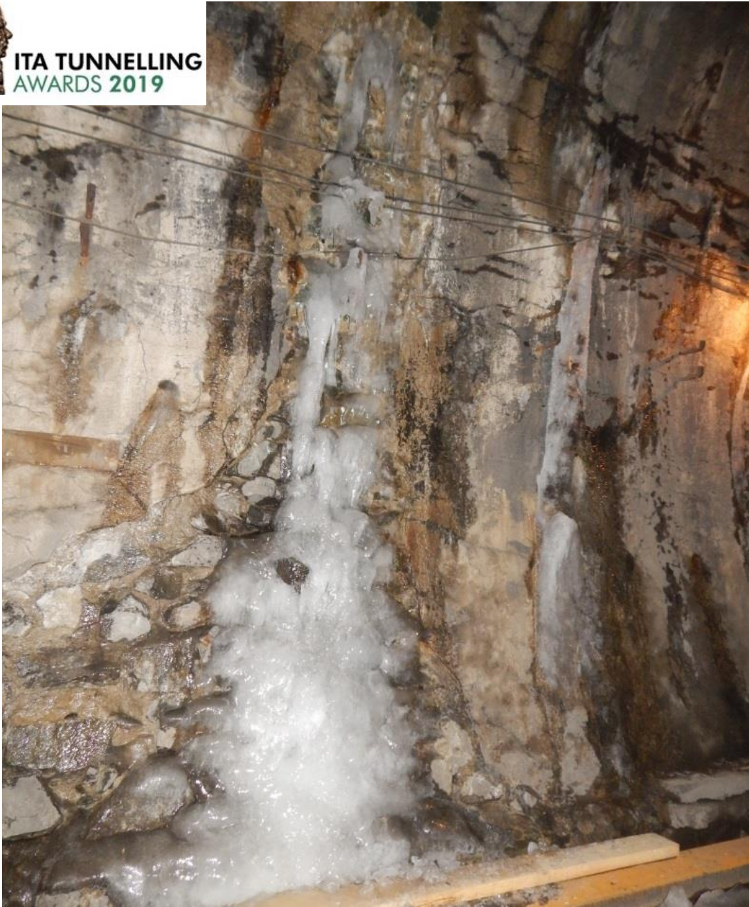
Aufeis formation in the tunnel
