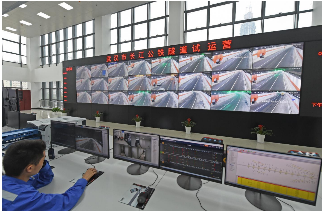
Tunnel Monitoring Center
