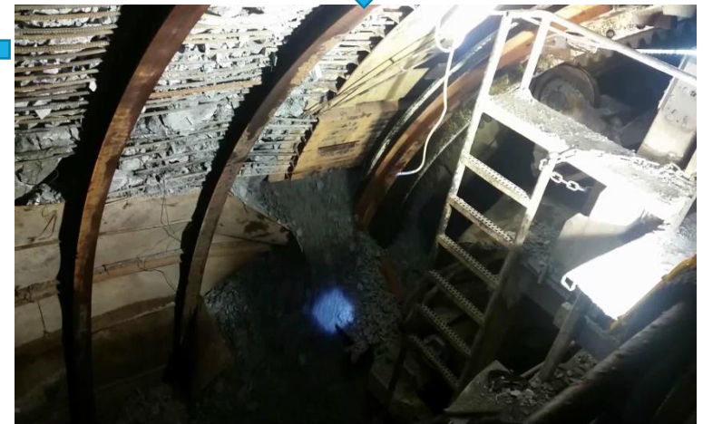
Fault fractured zone at K51+597
