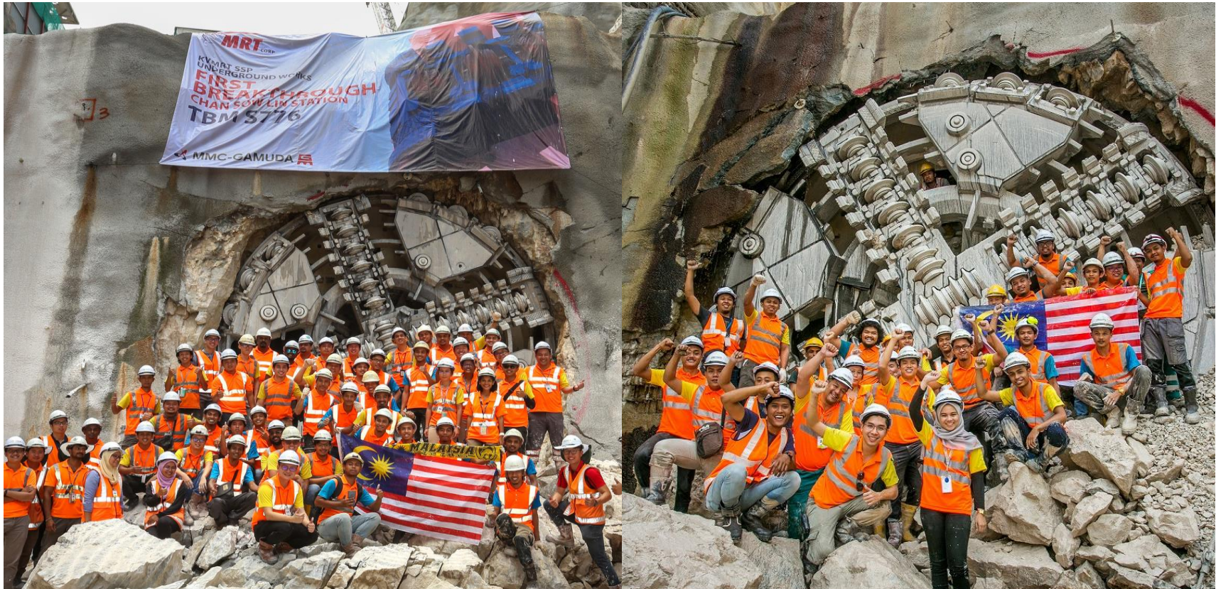
Breakthroughs of S-776 and S-777 – The first VD TBMs to Pilot Test our Autonomous TBM System
